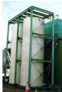
1999-2000: Middlesex University Ice Storage System – ammonia chiller
