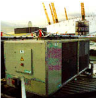
1999: McDonalds Education Centre, Millennium Dome – hydrocarbon chillers
