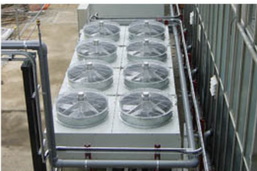
2001: Bath University Mechanical Engineering – air blast cooling system
